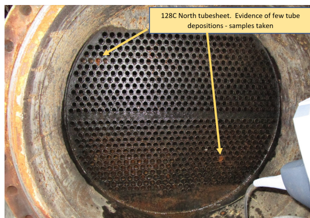
Figure 1. 128°C tube sheet from an ammonia plant inspection showing a hard deposit restricting the flow and heat transfer within the unit.
