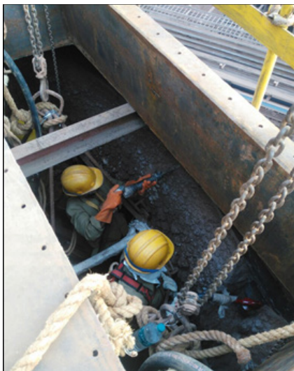
Figure 6. Wall Scale of the 1st Washer.
