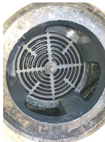
FIGURE 3: Compressor #7 valve at the time of opening.
