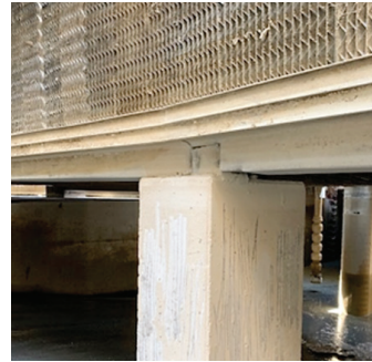
Image 2. Due to operational issues, the plant was unable to respond to the early deposit stress warnings. As a result, an iron-silica deposition event occurred which fouled the cooling tower and condenser and forced shutdown for remediation.
