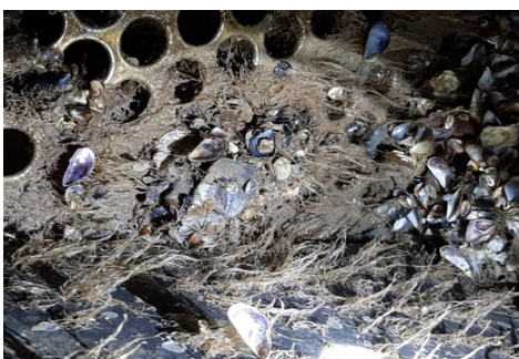
IMAGE 1: Macrofouling of condenser caused by mussels and debris
