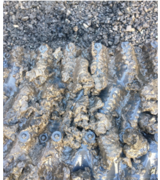
Phosphate-based deposit on the cooling tower fill which was removed from the tower.
