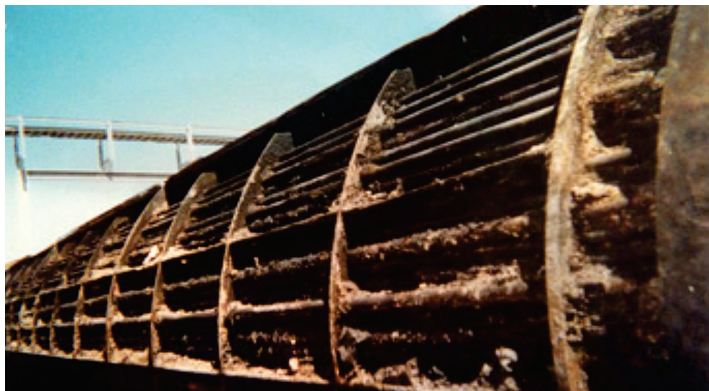
FIGURE 2: INTERSTAGE COOLER AFTER 5 YEARS ON LINE (RUN 1)
